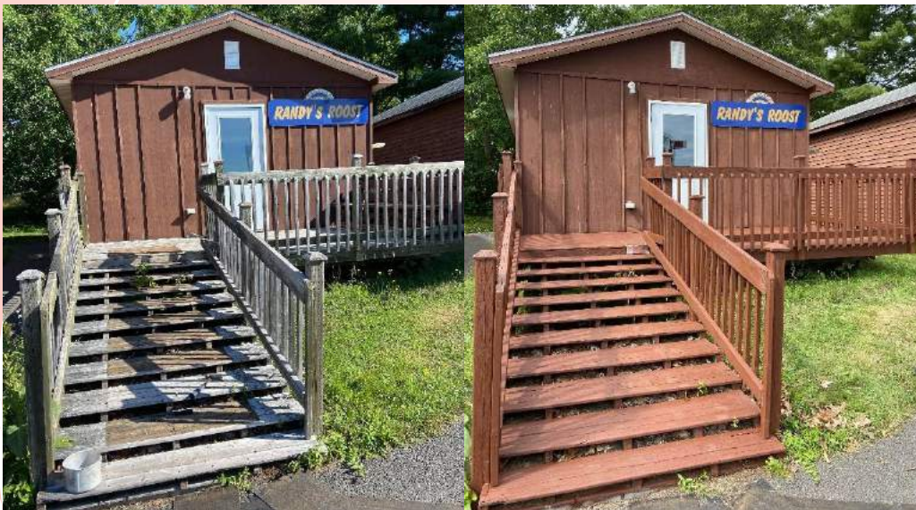
Before & after of one of Camp Rotary's 2020 summer renovations: re-staining the cabin decks!
